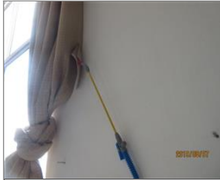
External photo(s) of the production unit(s) 7.7 Eye washing facility only have one head.JPG
