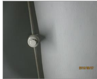
External photo(s) of the production unit(s) Smoke detector.JPG
