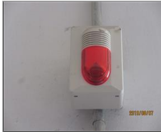
External photo(s) of the production unit(s) Fire alarm ring.JPG
