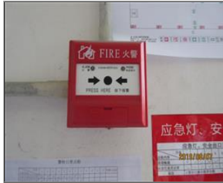
External photo(s) of the production unit(s) Fire alarm button.JPG
